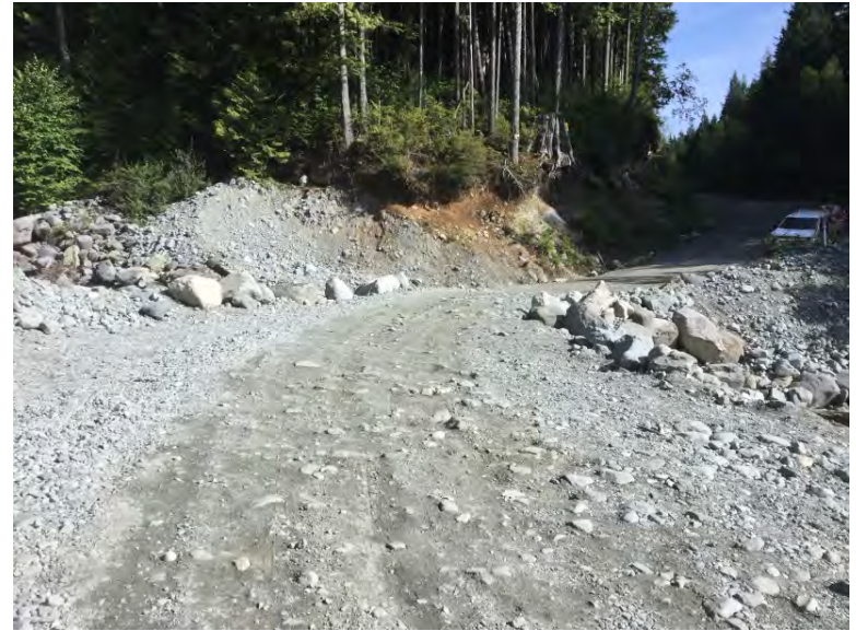
Road narrows substantially over culverts
